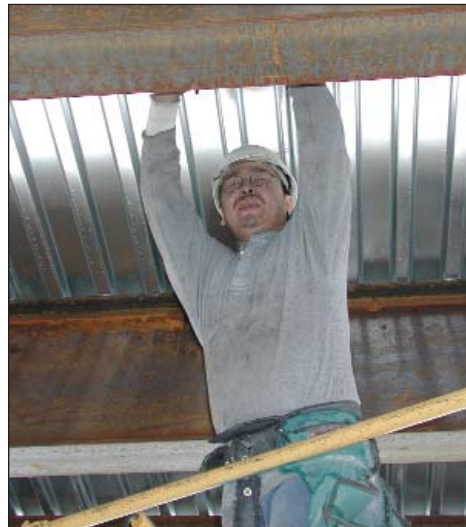
Native hire has been a priority on the construction of the Nonprofit Services Center
